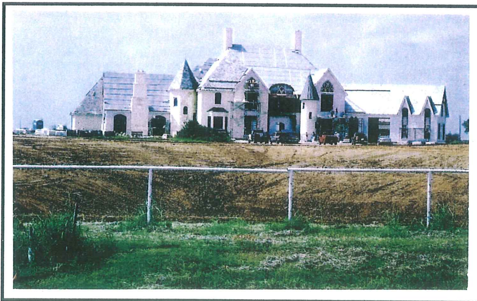
HOME ON THE RANGE — A reassuring sign for Sooner fans of football coach Bob Stoops is this house rising in northwest Norman on 36th Ave NW, just south of Indian Hills Road. The coach and his family will soon be moving into the place, whose construction cost some $3.3 million to $5 million (estimates vary).
